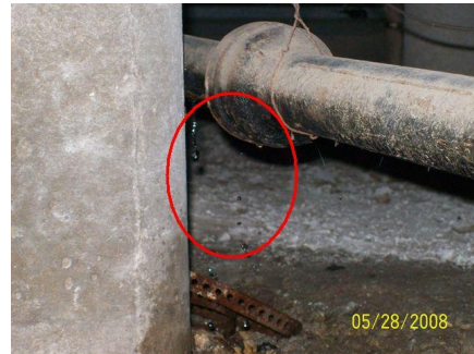
Leak under dining room floor (kitchen drain)
