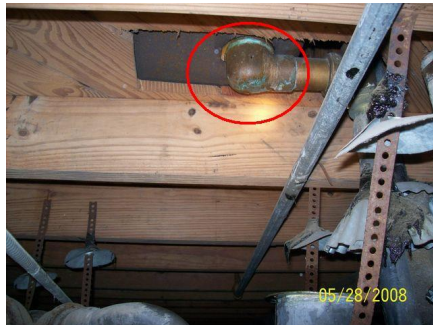
Leak observed under bath tub drain
