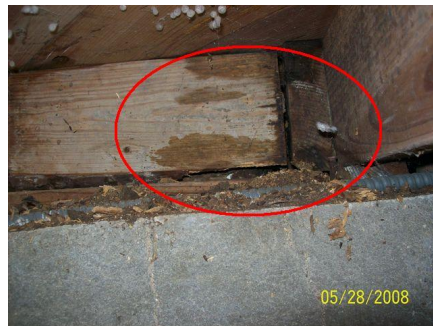
Damaged joist, back porch (from crawlspace)
