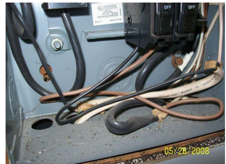
Bushings missing from panel entry points
